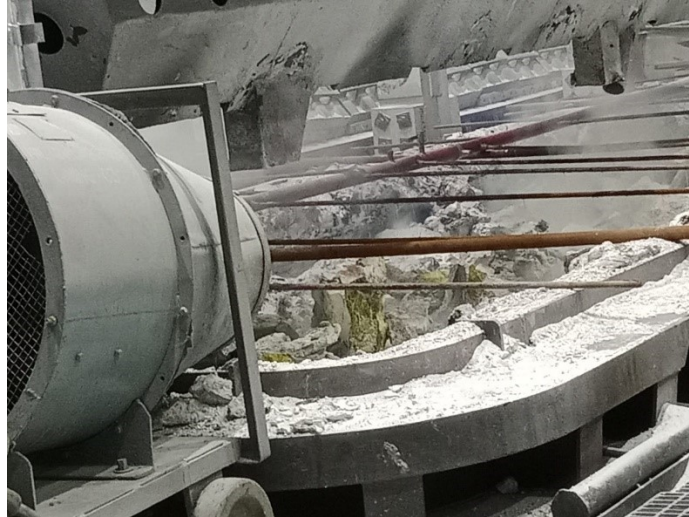
Figure 2. Water Spraying by water sprinkling system on a 235 kA pot.
